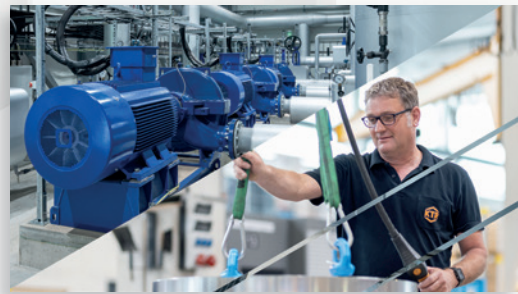
Pumps and compressors
